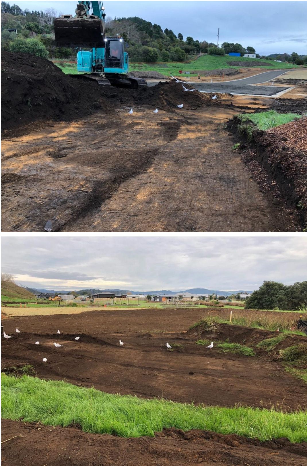
Figure 30. The two photos show stripping at the boundary of the reserve and new roading close to T11/1014 (top photo facing south bottom photo facing north)
